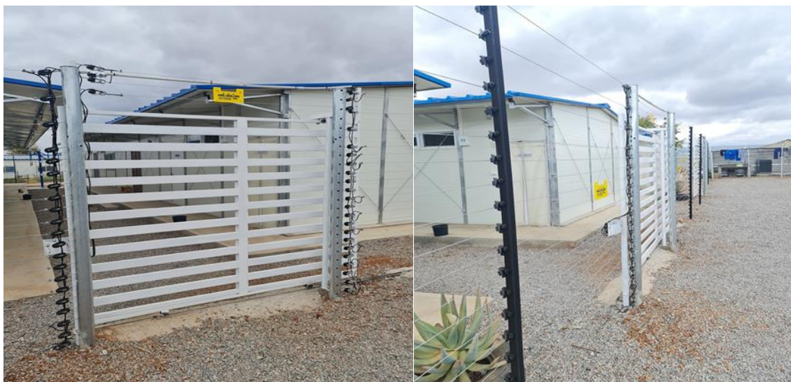
View of electrified fence and sliding gate
